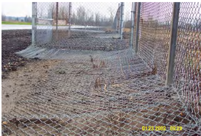
This photo shows an airport's perimeter fence with a 4-ft skirt attached to prevent animals from digging under it and to reduce washouts. (Photo courtesy PDX)
