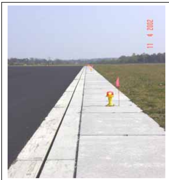
Figure 4. Slit type gutters, runway lights in concrete runway verge and snow flags at Twenthe airbase
