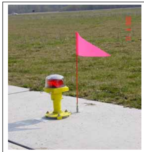
Figure 5. Runway light in concrete verge with snow flag acting as antiperching device
